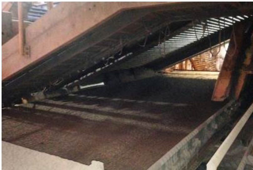
Figure 3.21. Conveyor belt for transport of fines sieved on double deck roller screen at Vargem Grande induration machine entrance.
